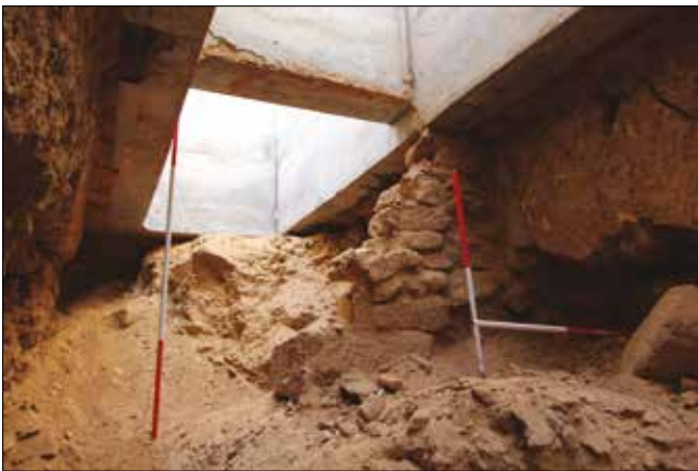
Plate 2. Cracks and holes on the northern wall of the descandary.
