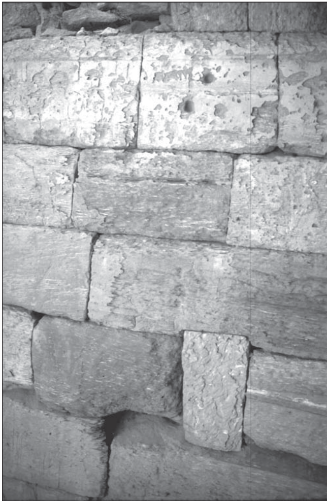
Plate 2. The chapel of pyramid BEG N 6: Southern chapel wall showing the the recent destruction of the surface and reliefs by wind erosion. (slide 9725)
