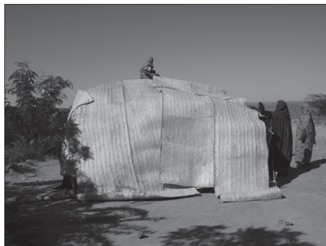
Plate 21. Climbing on the framework to secure the matting on the top of the structure.
